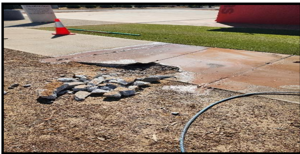
Removing and replacing of the footpath on Honour Avenue alongside St John Sub Centre.
